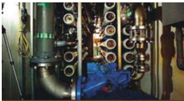
HW Process Technologies' patented Engineered Membrane Separation systems filter out the components of an aqueous stream by applying pressure and flow across a semi-permeable membrane. These high-performance systems can treat thousands of gallons of polluted water per minute.
